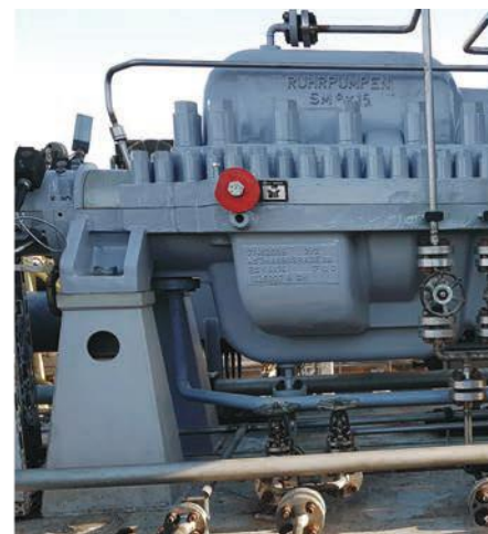
Pumping stations for seawater in Chile.
