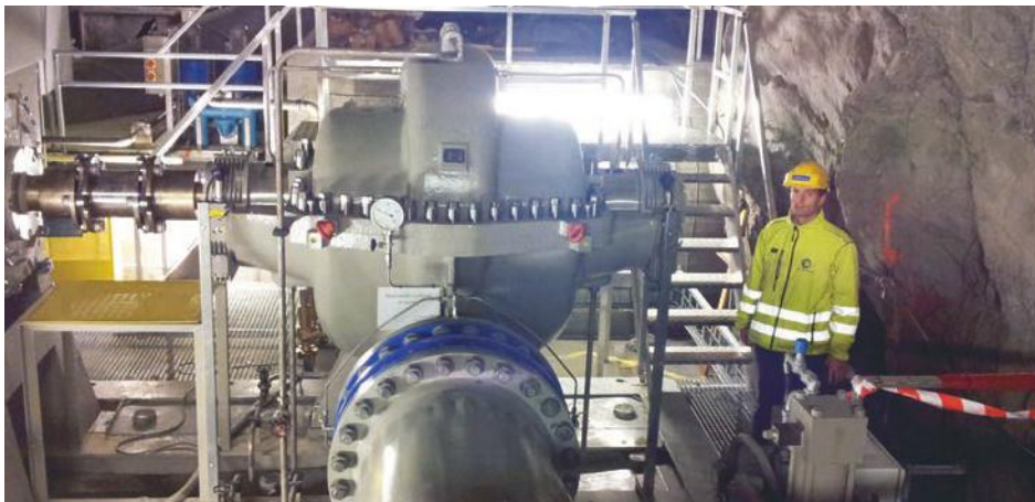
ZM pump installed in underground mine in Norway.
